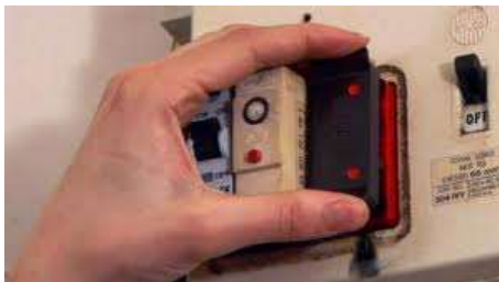
Older type fuse box
